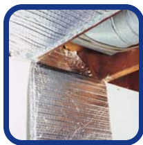
Crawl Space R-16.89
